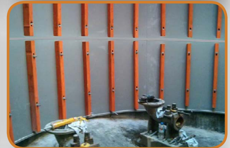
Continue Plastic Lining
